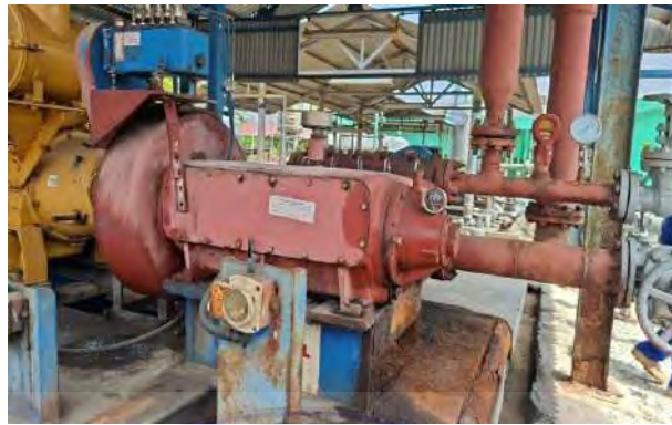
Gambar 3. 34 Pompa Water Injection Plant (WIP)
