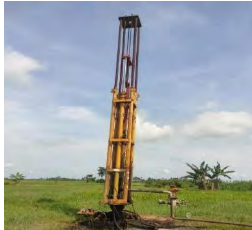
Gambar 3. 6 Hydraulic Pumping unit
