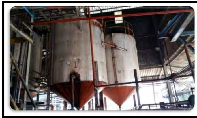
Gambar 3.14. Sand Trap Tank
