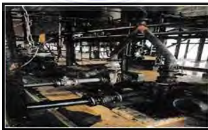
Gambar 3.19. Oil Transfer Pump
