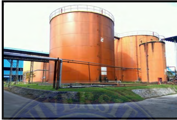
Gambar 3.20. Oil Storage Tank
