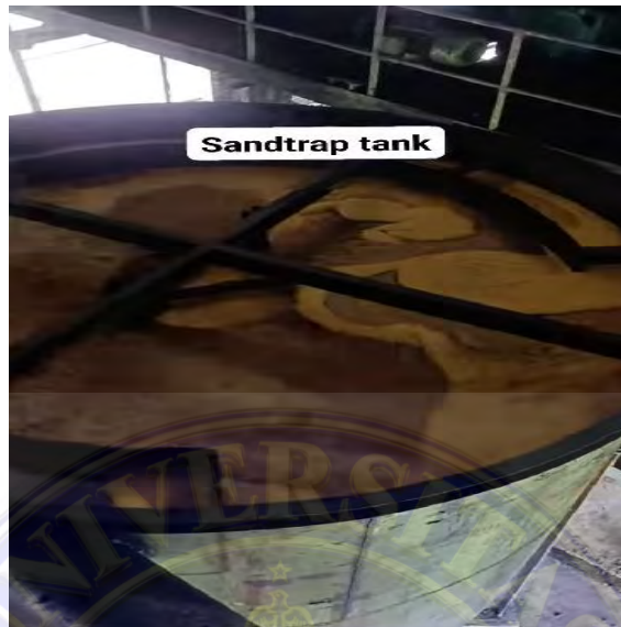
Gambar 3. 19 Sand Trap Tank
