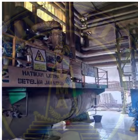
Gambar 3. 42 Back Pressure Vessel
