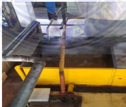
Gambar 3. 25. Water Phase Tank
