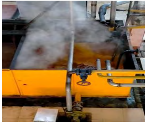
Gambar 3. 24. Oil Collecting Tank
