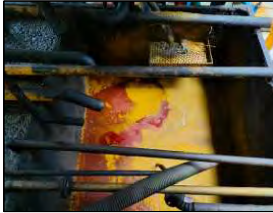
Gambar 3.27 Oil collecting tank
