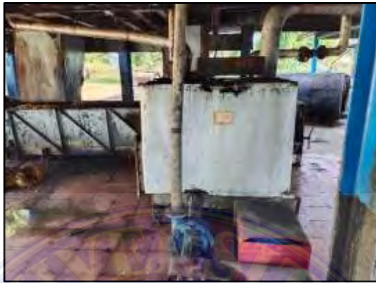
Gambar 3.13 Crude oil tank 1
