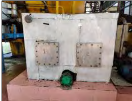
Gambar 3.17 Crude Oil Tank
