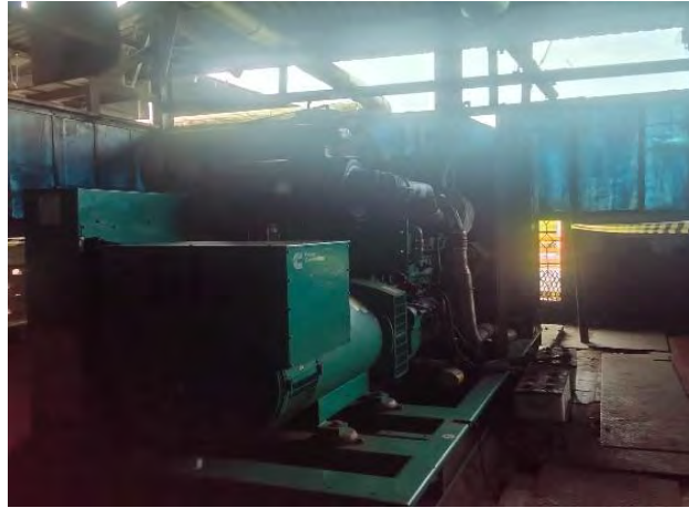
Gambar 3. 56 Diesel Engine (Genset)
