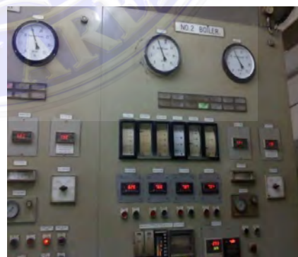
(b) Ruang kontrol Boiler
