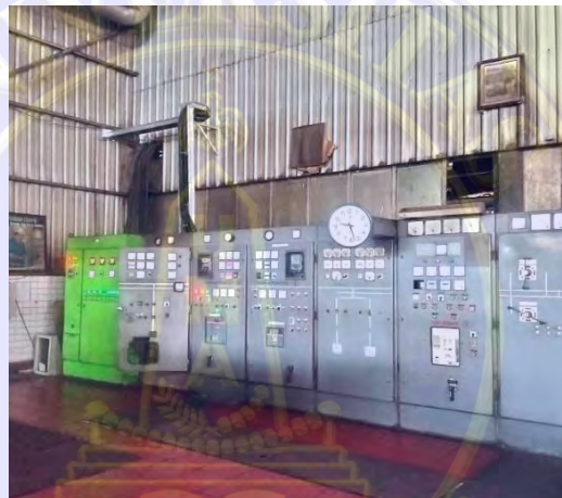
Gambar 3. 58 Main Switch Distribution Board
