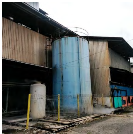
Gambar 3. 65 Feed Water Tank
