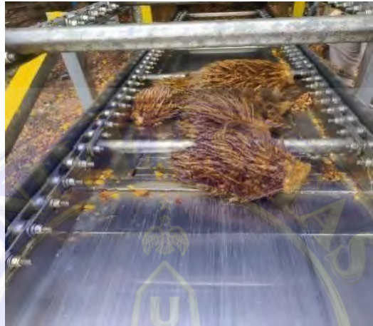
Gambar 3. 26 Empty Bunch Conveyor
