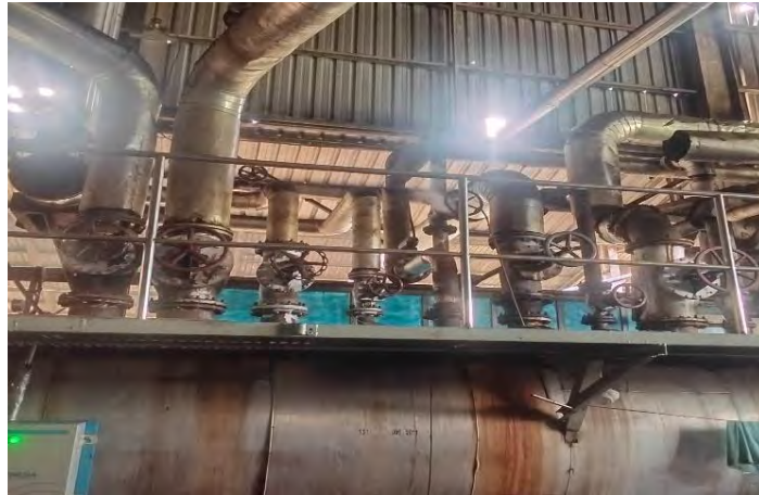
Gambar 3. 56 Back Pressure Vessel
