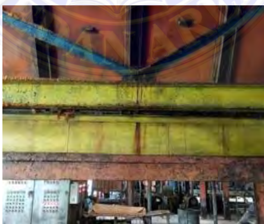
Gambar 3. 21 Under Thresher Conveyor
