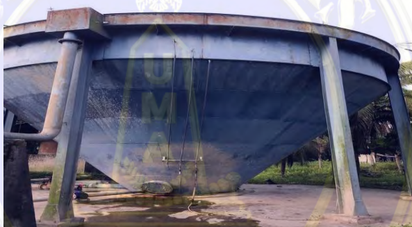
Gambar 3.51. Water Clarifier Tank
