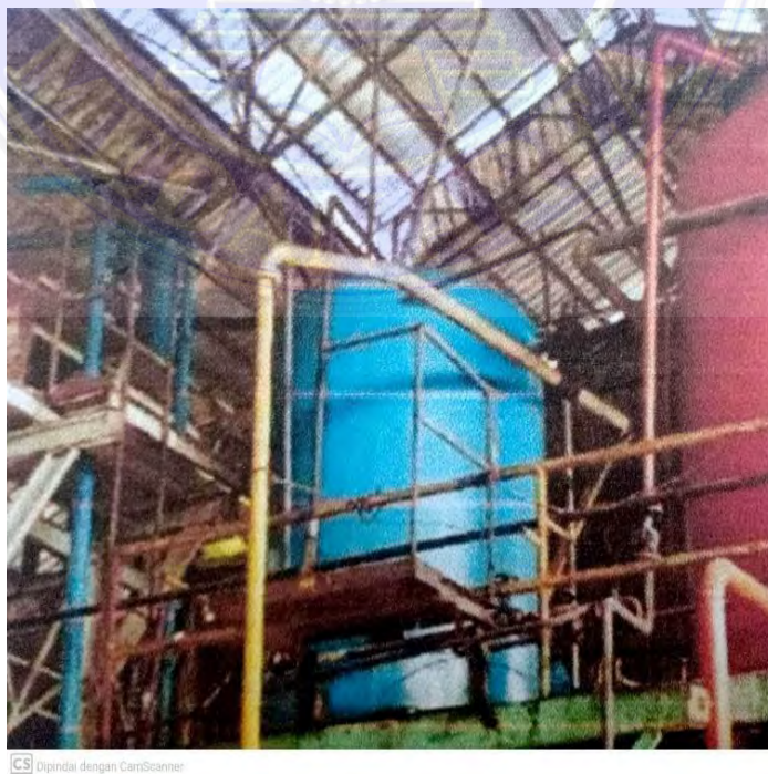
Gambar 3.30. Hot Water Tank
