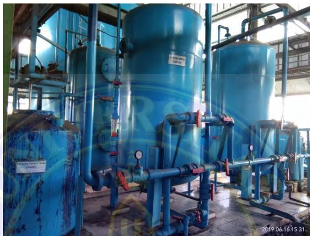
Gambar 3.55. Anion Tank dan Kation Tank
