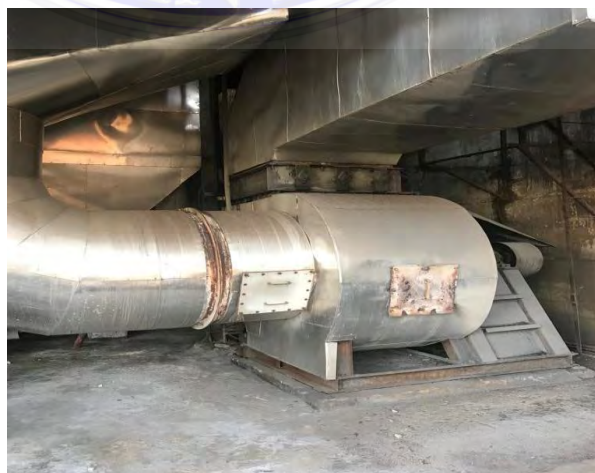
Gambar 3.47. Induced Draft Fan
