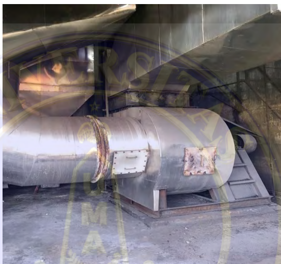
Gambar 3. 62 Induced Draft Fan
