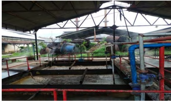
Gambar 3.32. Bak Penampung Sludge (Fat Fit)
