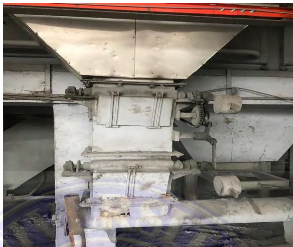
Gambar 3.48. Damper Dust Collector
