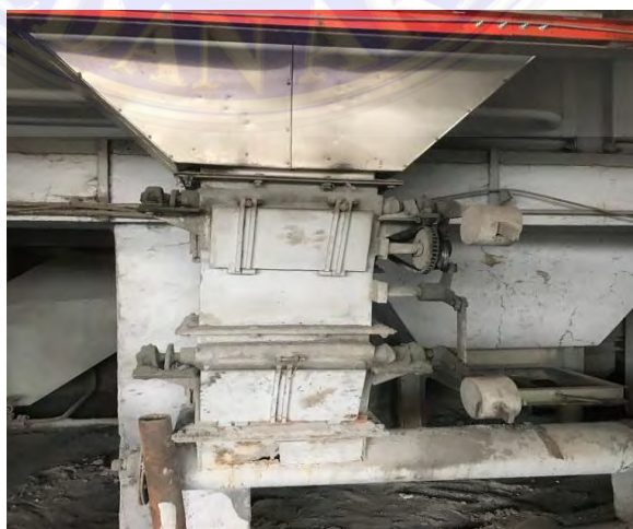
Gambar 3. 63 Damper Dust Collector
