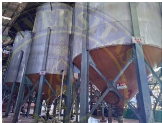
Gambar 3. 29 Continuous Settling Tank (CST)
