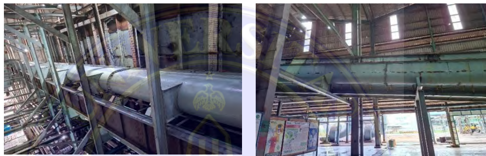
Gambar 3. 42 Cage Breaker Conveyor
