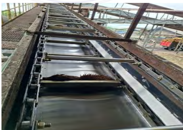
Gambar 3. 20 Empty Bunch Conveyor
