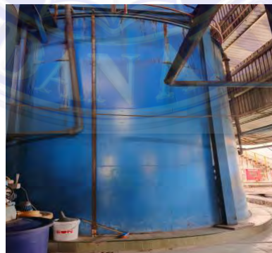
Gambar 3.58 Feed Water Tank
