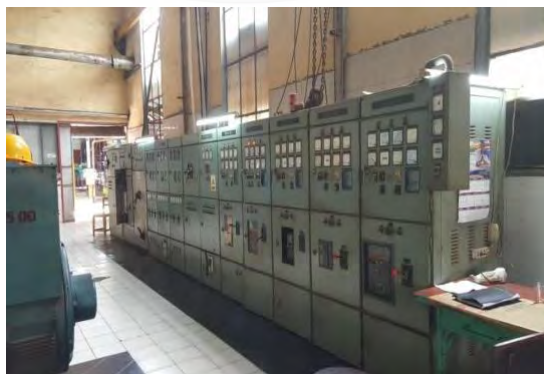
Gambar 3.50 Main Switch Distribution Board ( Panel Kontrol Utama )
