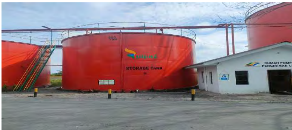
Gambar 3.20 Oil Storage Tank
