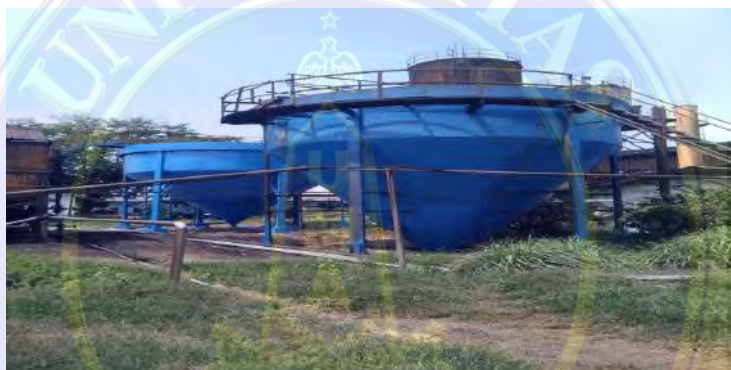
Gambar 3.23 Tangki Pengendapan ( Clarifier tank )
