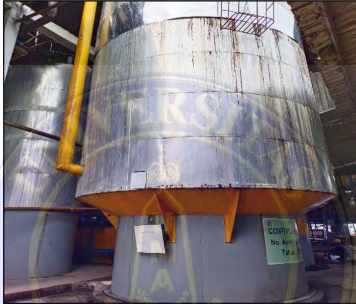
Gambar 3. 25 Continuous Settling Tank
