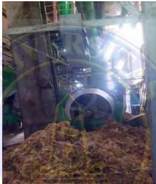
Gambar 3. 14 Cake Breaker Conveyor (CBC)
