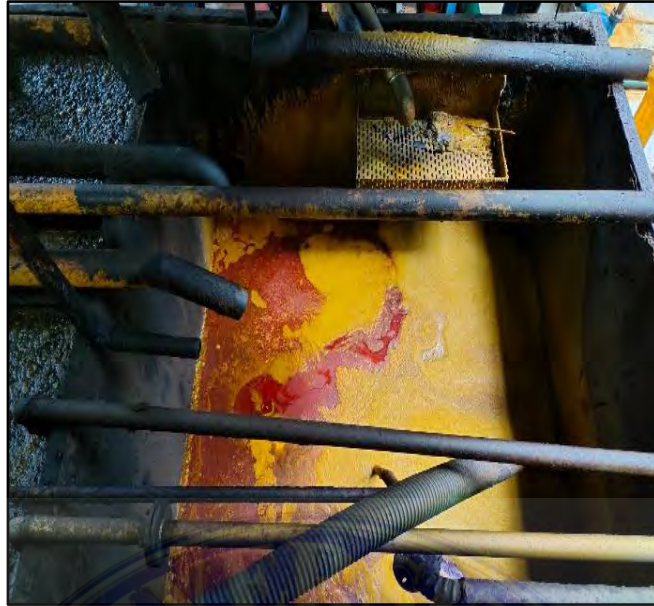
Gambar 3. 33 Oil Collecting Tank
