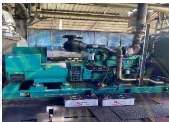
Gambar 3.56 Diesel Engine (Genset)
