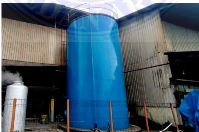
Gambar 3.64 Feed Water Tank
