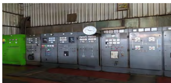
Gambar 3.57 Main Switch Distribution Board (Panel Kontrol Utama)
