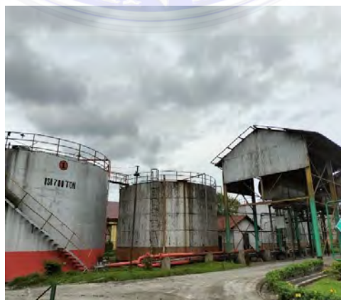
Gambar 3.16 Oil Storage Tank
