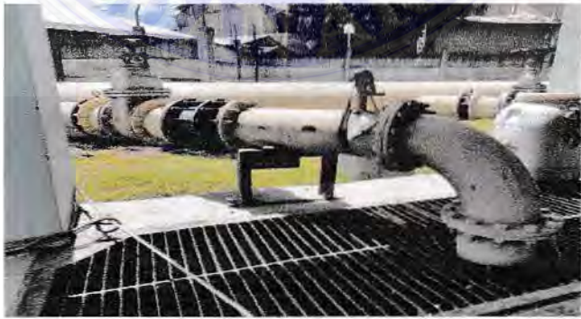
Gambar 3.3. Raw Water Pump
