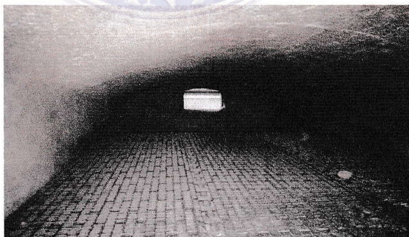
Gambar 3. 1. Ruang Bakar Boiler
