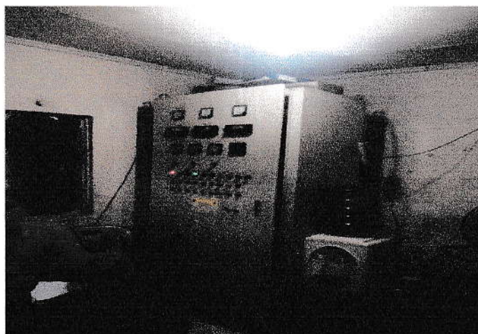
Gambar 3. 7. Panel Kontrol Boiler
