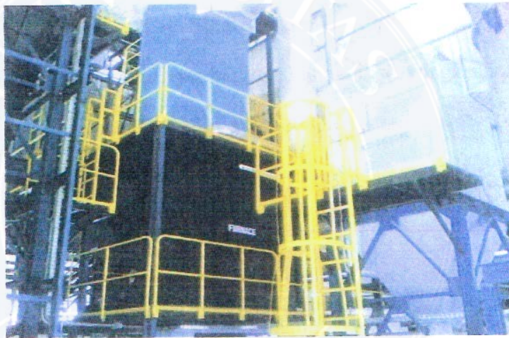
Gambar 2.9. TOH (Thermal Oil Heater)
