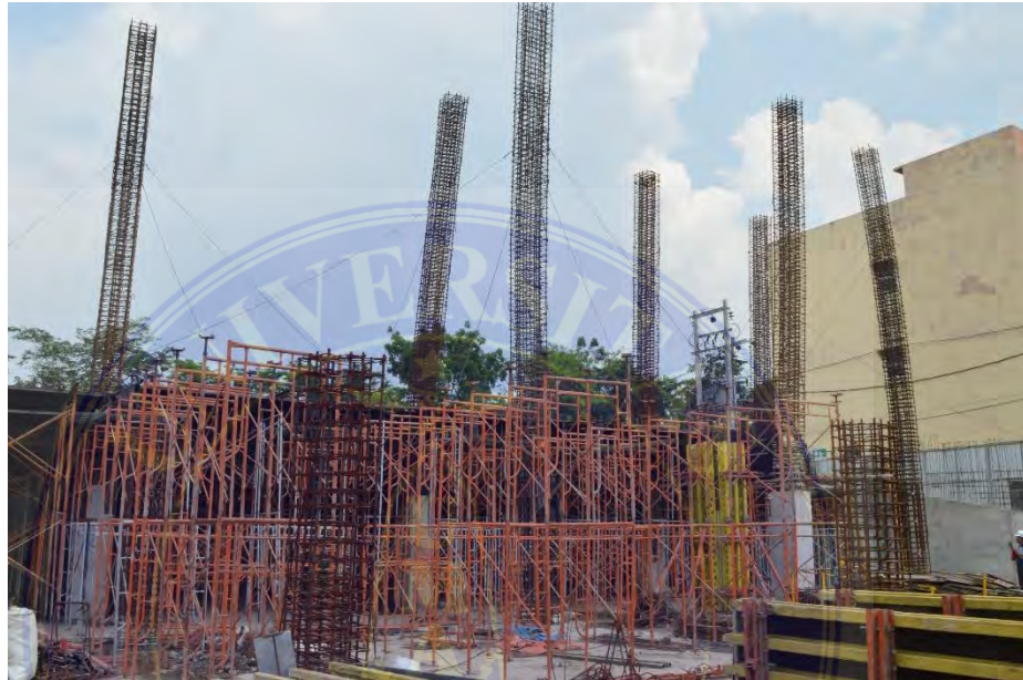
Gambar 2.11 Perancah jenis baja ( scaffolding ) (Sumber: Dokumentasi proyek The Manhattan Mall and Condominium)
