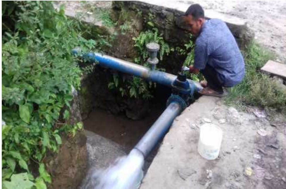
Wash Out Pipa Transmisi
