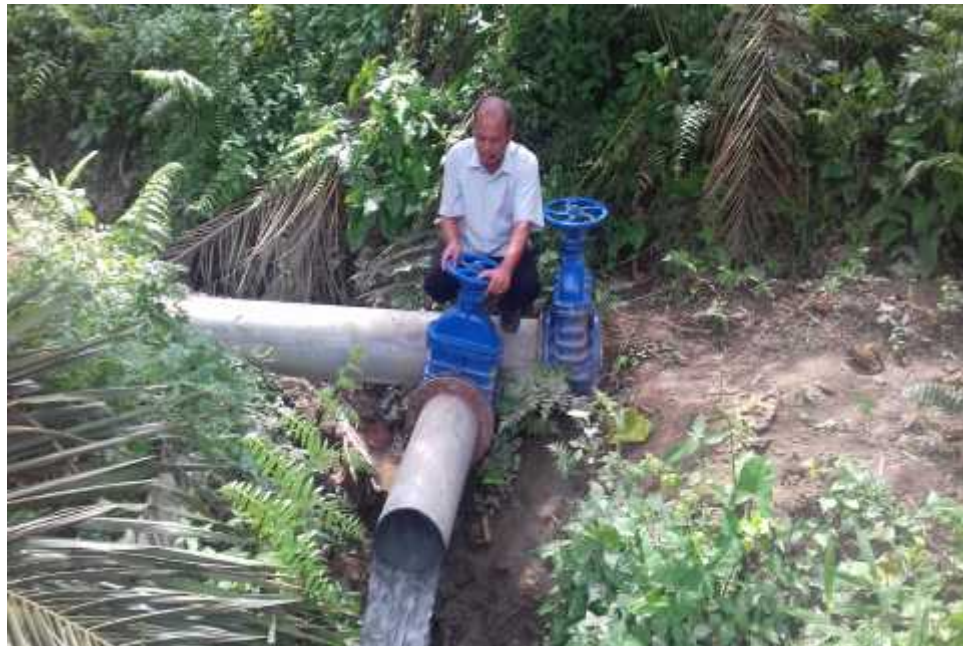
Wash Out Pipa Transmisi
